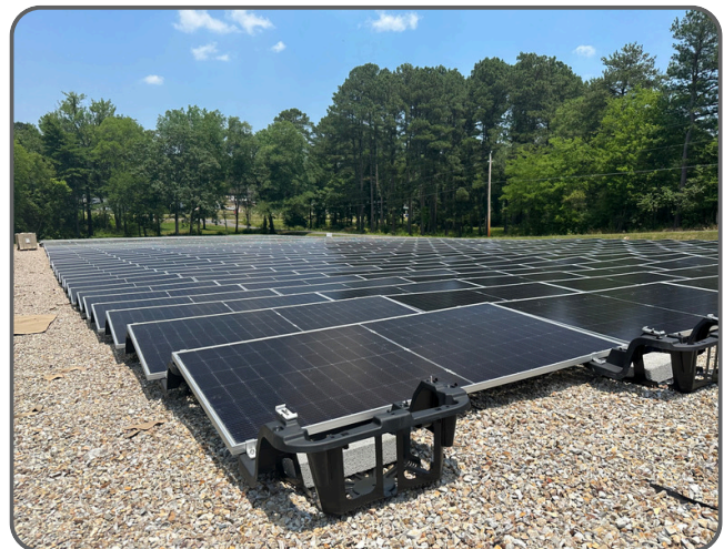
Hotsprings, AK 390 kW (Gravel)
